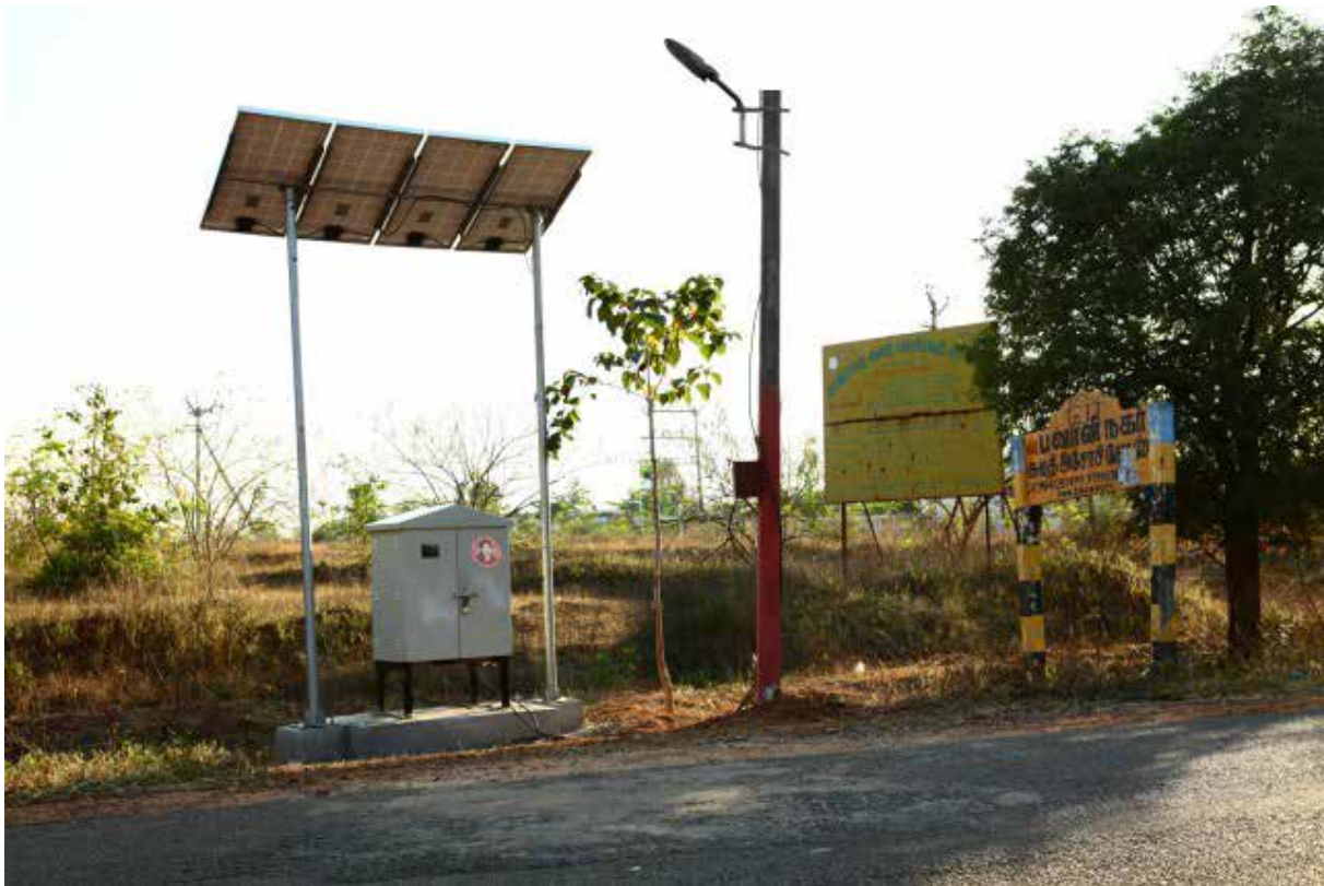
FIGURE 10: Solar street lighting
